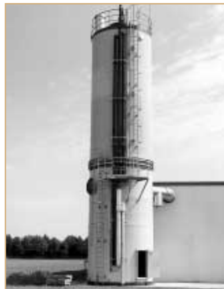
Moving Bed Trickling Filter (foto: RCL Heerenveen)
